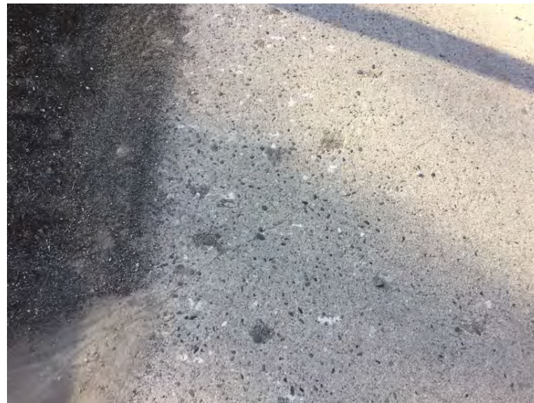
Hairline cracks noted on top of 2 deck panels
