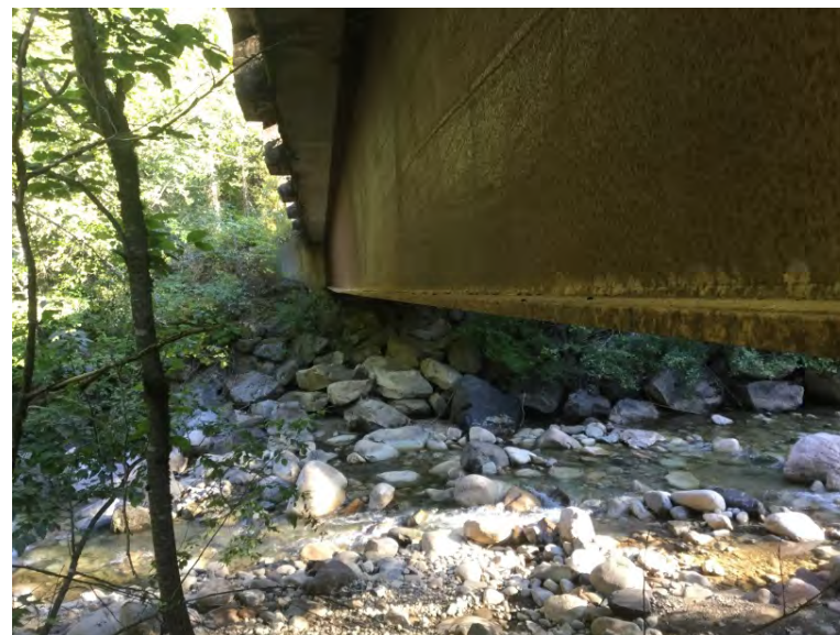
Sag in girders, downstream girder shown above
