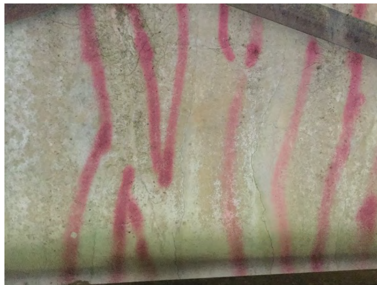
Hairline cracks in right bank ballast wall
